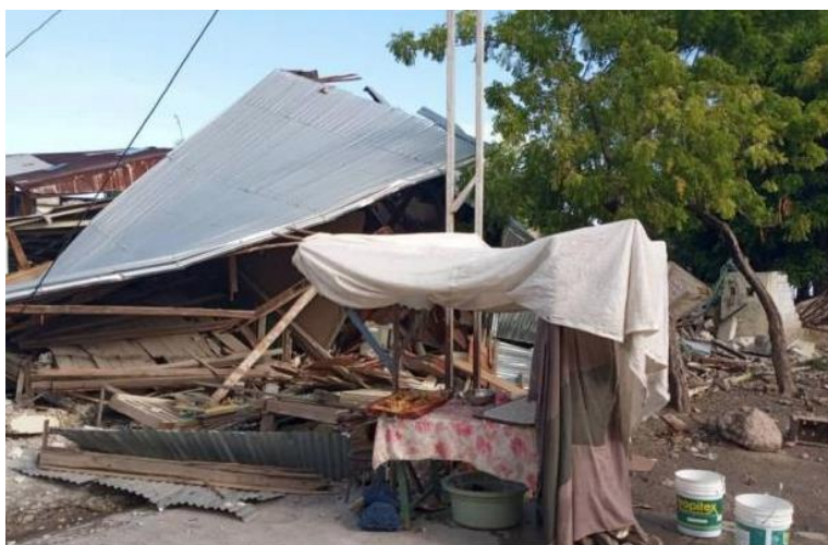
Buildings damaged by the earthquake in Haiti, August 2021.
